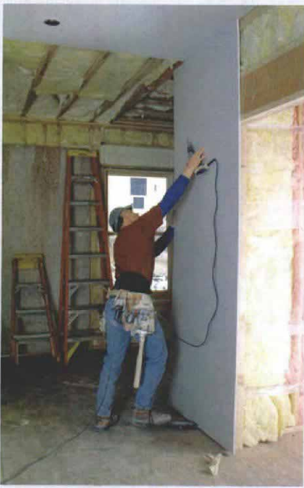
Steady the sheet with one hand until it's held tight to the ceiling with foot pressure.
